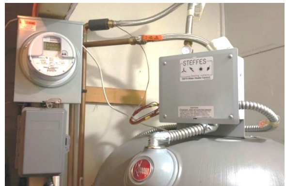
Steffes GETS controller on a customer's water heater. Courtesy of Lake Region Electric Cooperative.
